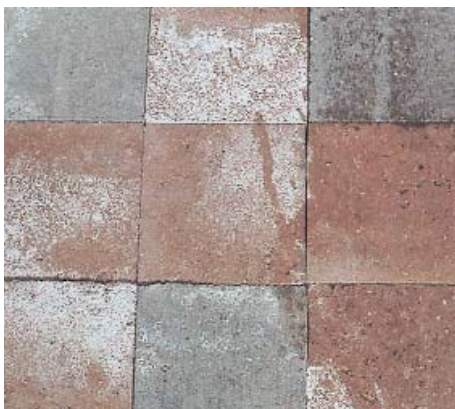
Block paving showing efflorescence
